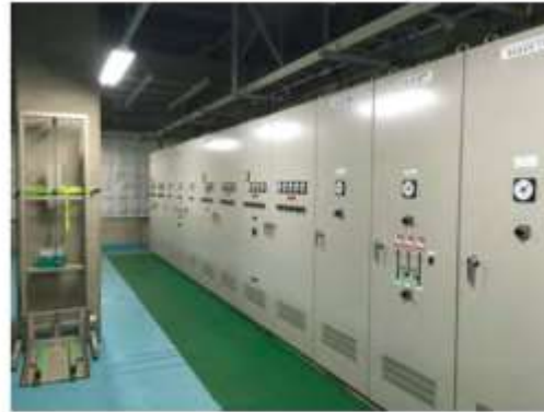
High voltage power receiving panel
